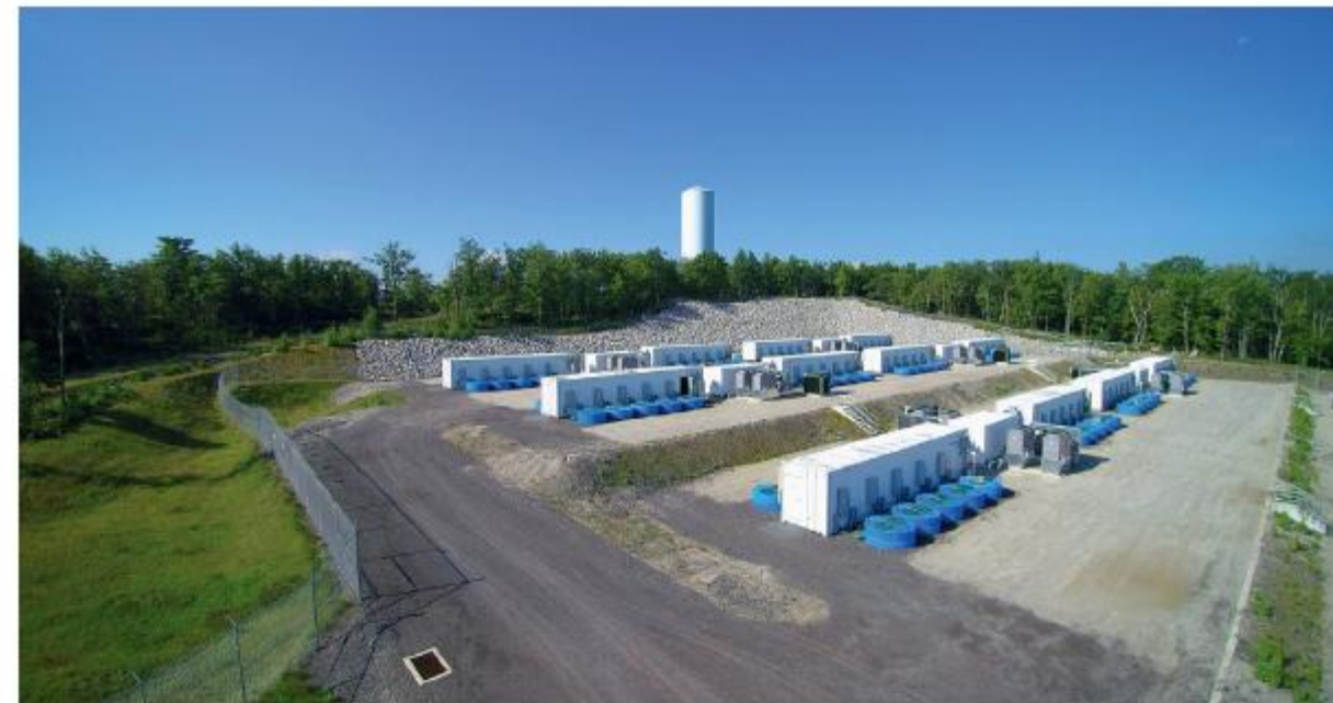
FIGURE 10.4 20 MW flywheel frequency regulation plant. (Source: Courtesy Beacon Power LLC.)
