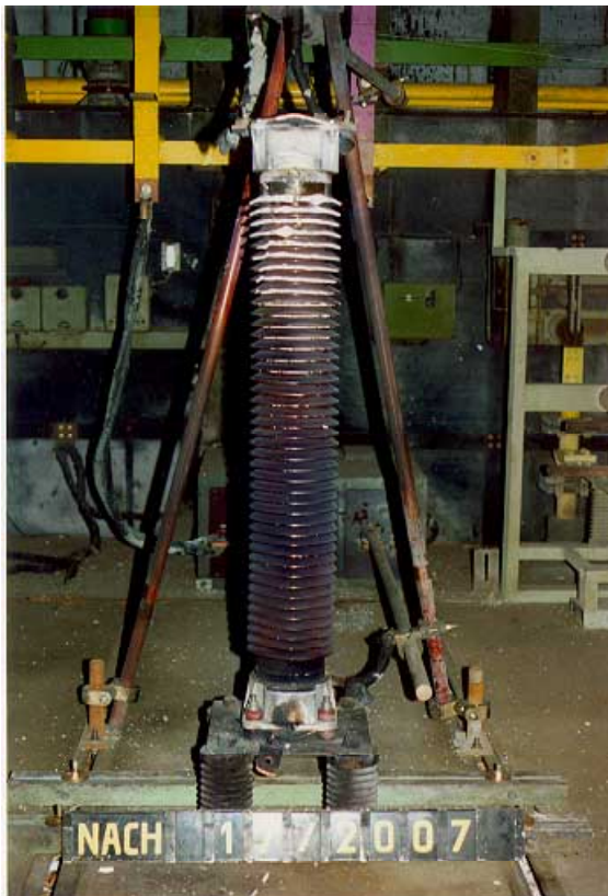
Fig. 22: Porcelain housed arrester after pressure relief test with rated short-circuit current (63 kA, 200 ms). With the exception of some sheds which were broken the housing remained intact.
